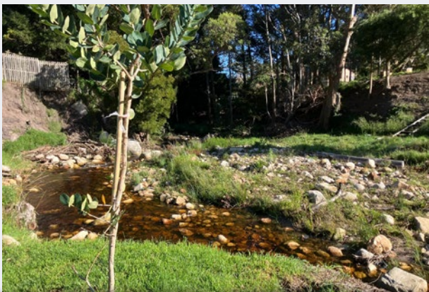
Alien vegetation on an in-channel bar led to accumulation of sediments such that the main channel of the river was deflected into the secondary channel, causing severe bank and bed erosion, that necessitated the installation of groynes and the removal of excess sediment from the bar.
