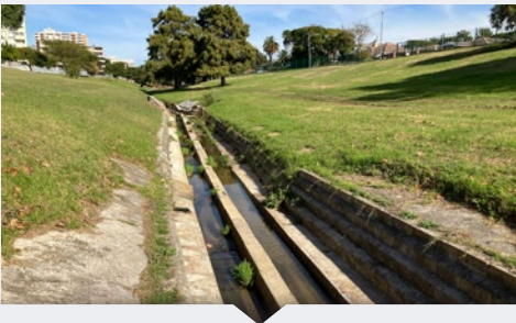
Low flow section of Elsieskraal River canal (Cape Town), designed to speed up flows and prevent sedimentation
